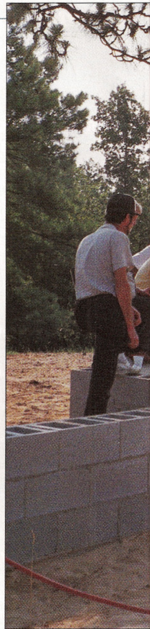
A basic understanding of how homes and other buildings are constructed will enhance your termite inspections and applications. One way to do this is to visit a construction site at various stages to learn how new homes are built.
