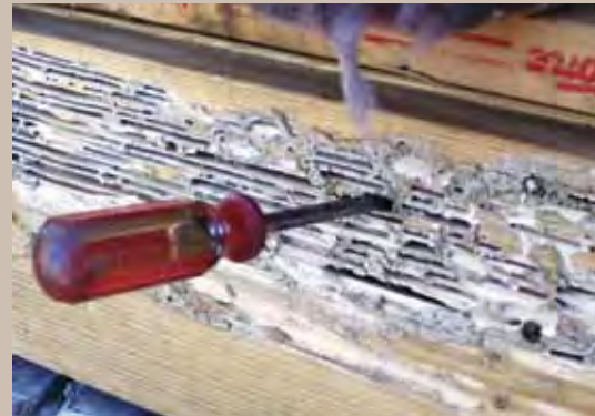
The National Pest Management Association (NPMA) estimates termites cause more than $5 billion worth of structural damage per year.
